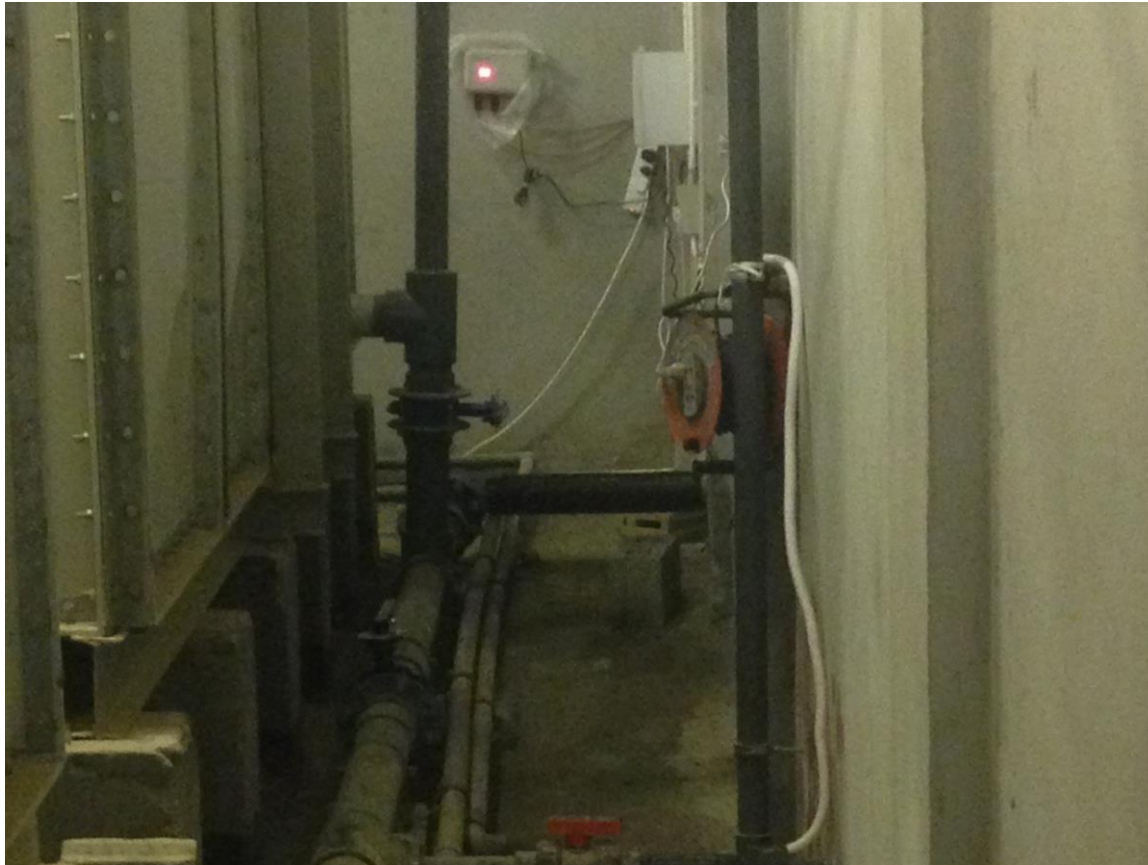
IE8 SW Model installed in the 4” outlet pipe of the water storage tank with 1 set of coil of 85 loops.
