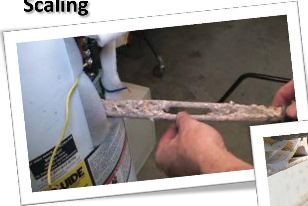
Scaling on water heater
