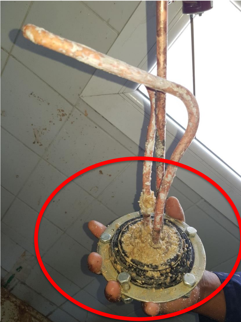
Before treatment Heating Element covered with scaling and corrosion deposits (9 th March 2018)
