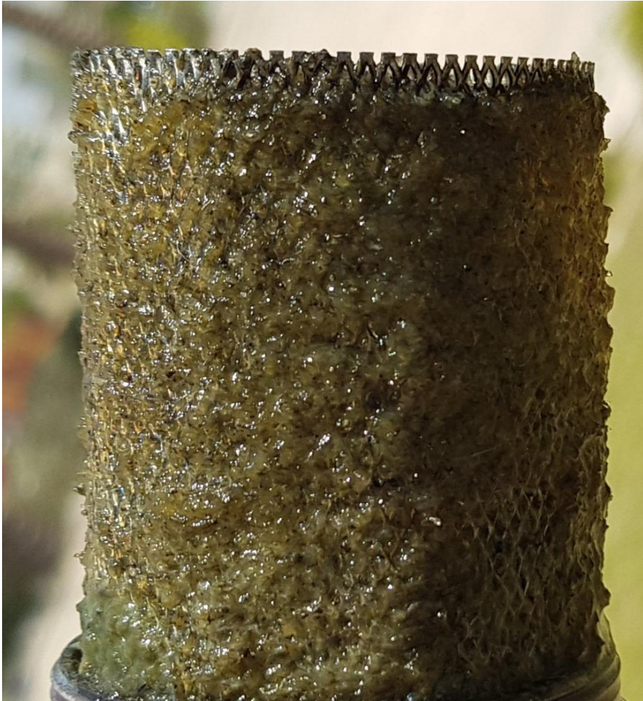
Before Installation, 20 th March 2019 Thick and Greenish microorganism covering whole strainer
